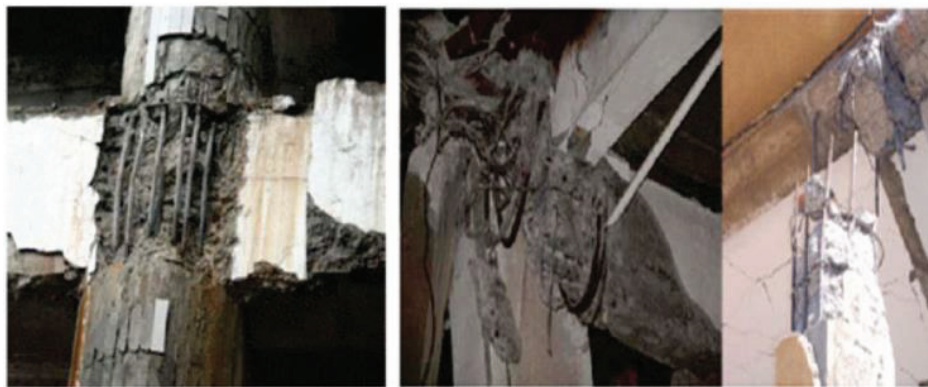
Fig. 30: Beam–Column Joint Failure.
